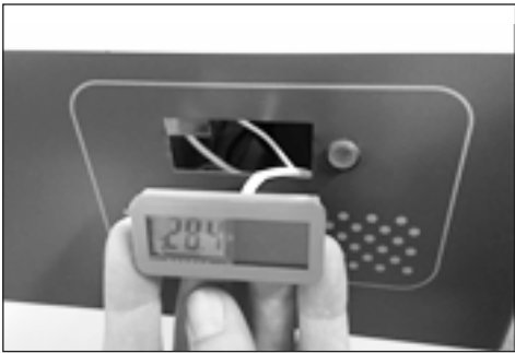
6. Temperature monitor is loose from cabinet.
