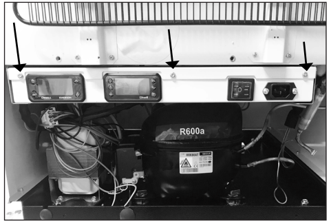
13. Remount junction box cover.
