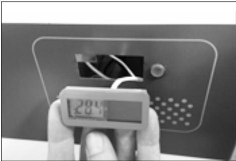
6. Temperature monitor is loose from cabinet.
