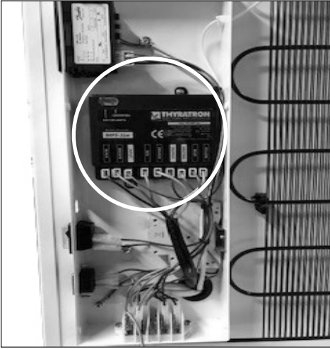
1.The controller is placed in the bottom
