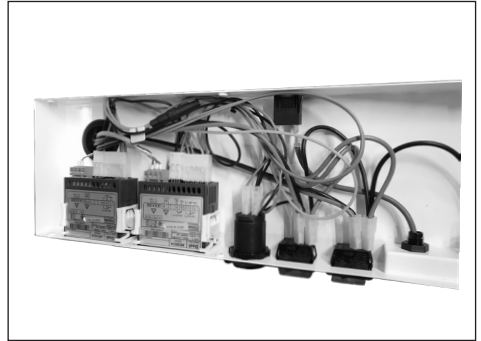
It's the same procedure that needs to be done for both of the thermostats
