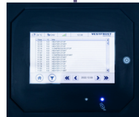
Remote alarm logs
