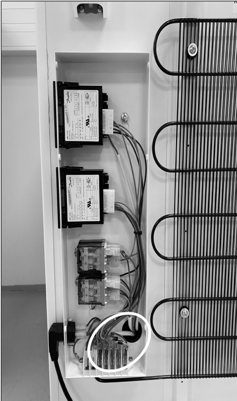
1. Junction Box and connection board
