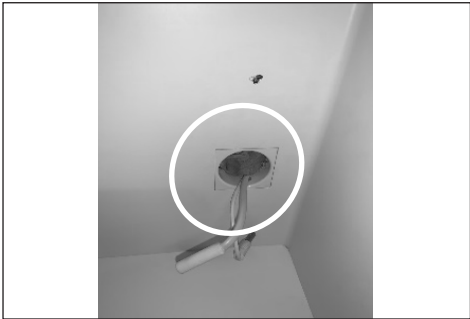
9: IMPORTANT! When re-mounting the new thermostat remember to properly seal the wire feed-through in vaccine compartment
