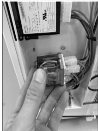
5. The relay is now loose.
