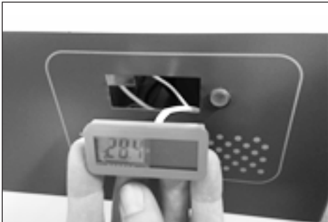
8. Temperature monitor is loose from cabinet
