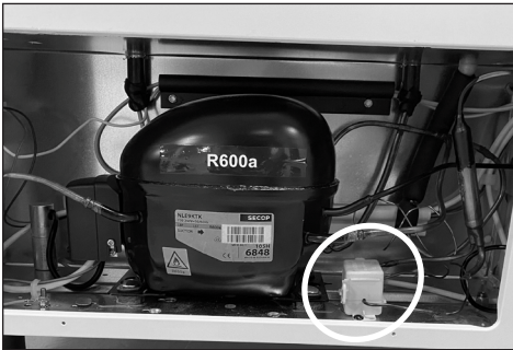
Valve to be replaced
