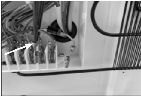
4. The diode is loose from the connection board
