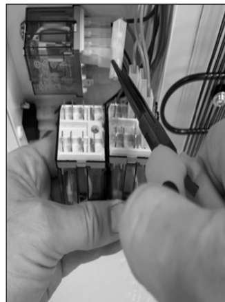
7. Use a plier to unmount and remount the lugs in the new relay.
