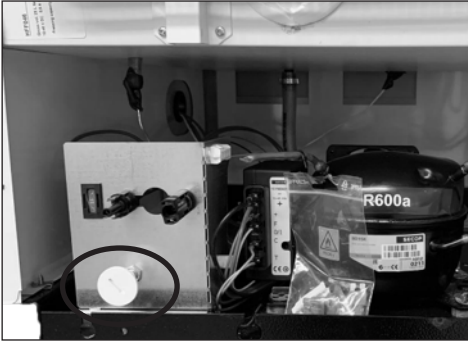
The thermostat is placed in the left corner of the compressor compartment
